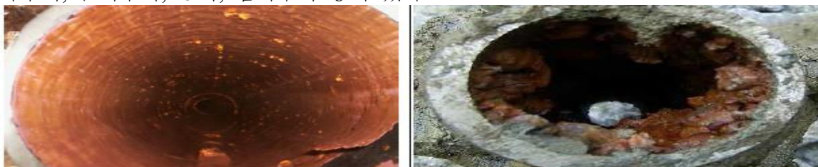
Fig. 3 Internal Corrosion of Pipe
