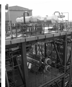
Figure 5. SCWO commercial plant for wastewater from TPA manufacturing plant
